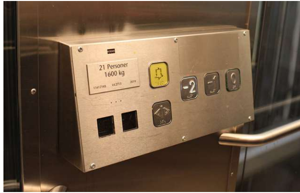
Figure 14: Operating elements inside E3 and E4
