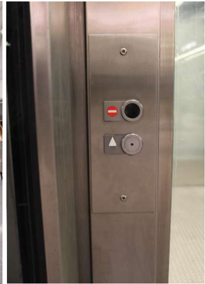
Figure 144: Operating elements elevator platform M3 outside
