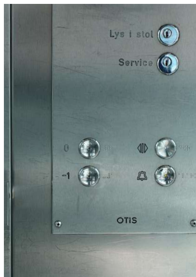
Figure 51: Operating elements inside E2 on platform M1/M2
