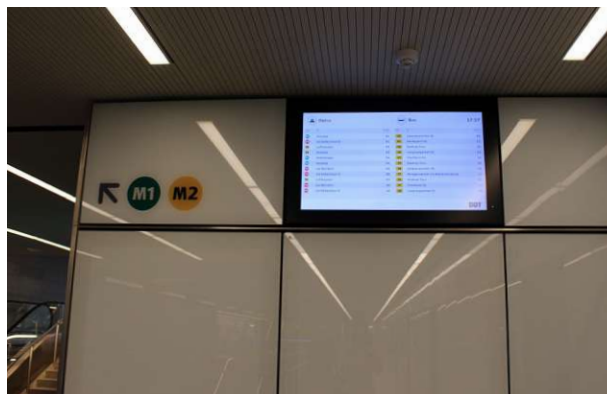
Figure 61: Monitor on passage level
