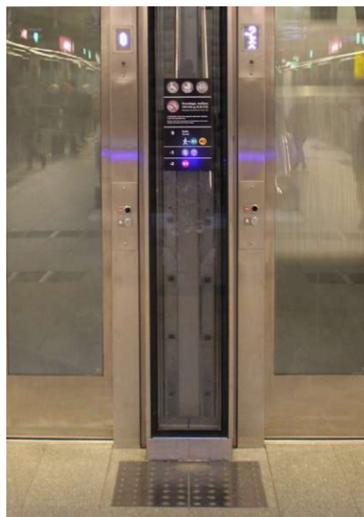
Figure 86: Operating elements outside the elevators on platform M3
