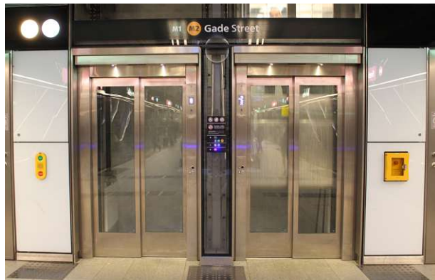
Figure 15: Elevators on platform M3
