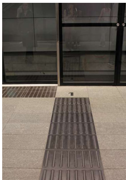
Figure 16: TWSI on platform M3
