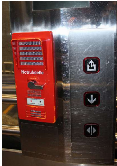
Figure 113: Operating elements inside E5
