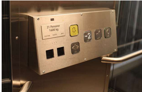
Figure 87: Operating elements inside E3 and E4
