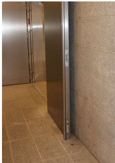
Figure 79: Open door posing an obstacle
