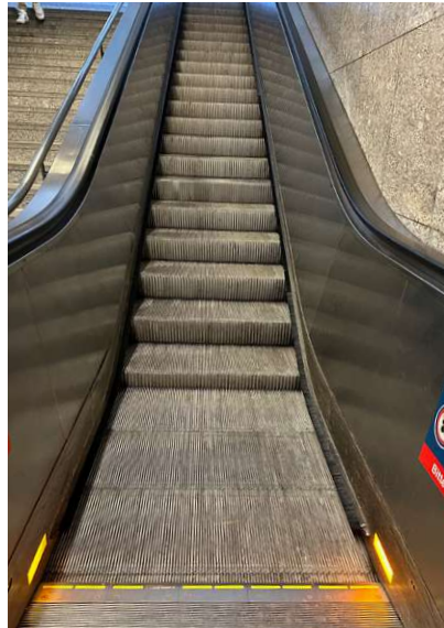
Figure 97: Escalators at Längenfeldgasse station
