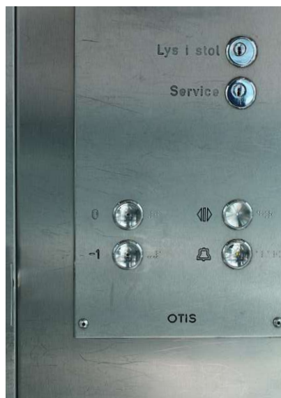
Figure 67: Operating elements inside E2 on platform M1/M2
