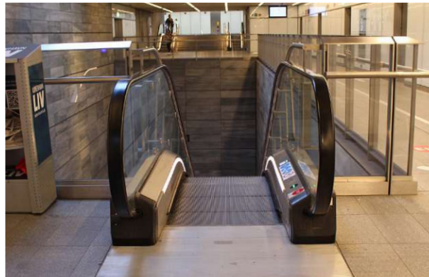
Figure 43: Escalators on passage level
